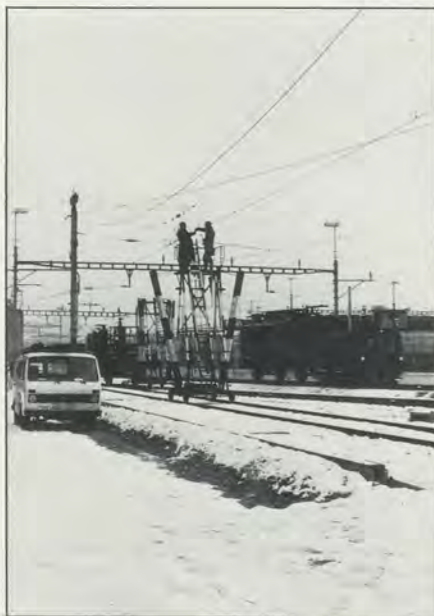
Assembly and control of specific connections, employees of Swiss Federal Railways at Zurich main station.
